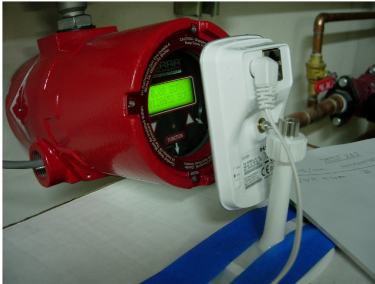
Figure 3. Gas Meter with Data Bus connected to DAQ and Webcam for Remote Reading
