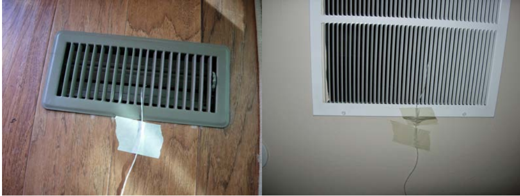
Figure 14. Temperature sensors in floor register and return grille
